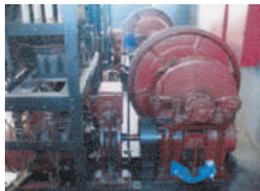
Original DC Motor Generator Set
