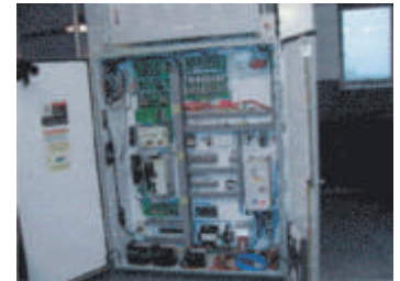
Upgraded Microprocessor Controller
